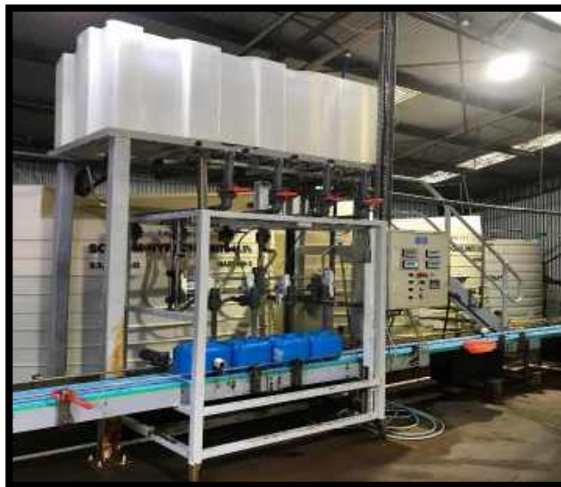
SODIUM HYPOCHLORITE FILLING PLANT FORMULA'S MODERN CHLOR/ALKALI STORAGE AND FILLING EQUIPMENT (110,000L STORAGE CAPACITY)
