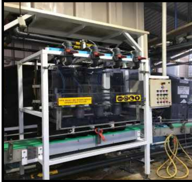
HYDROCHLORIC ACID FILLING PLANT (40,000L STORAGE CAPACITY)
